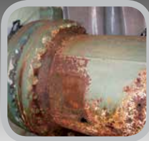
Pipe Before Repair
